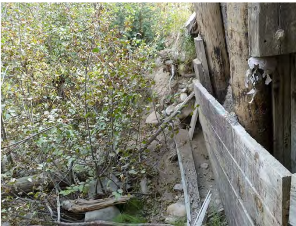
Figure 1-15: Downstream camp end wingwall rotating outwards.
