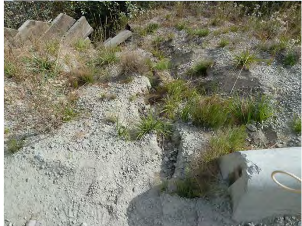
Figure 1-8: Erosion channel, downstream side of camp end approach embankment.
