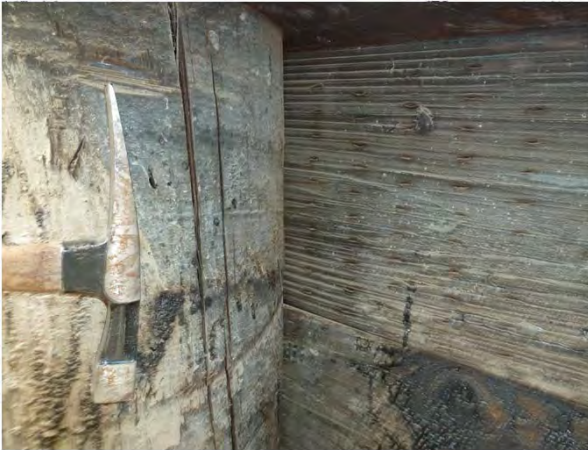
Figure 1-19: Split in pile 1 woods end.
