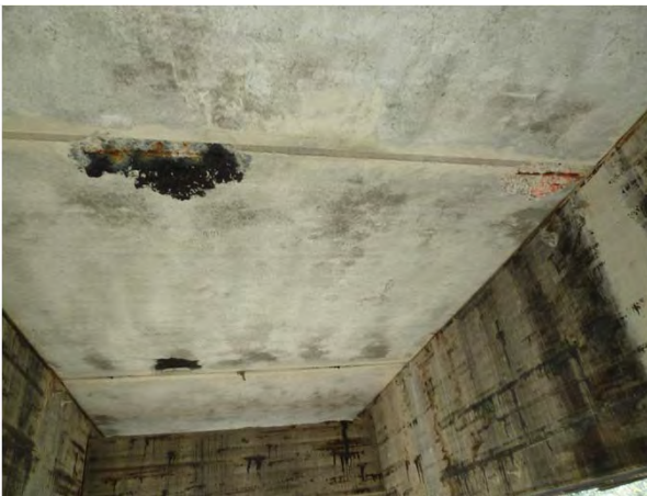
Figure 1-9: Typical underside of deck condition, note spalling at joint.
