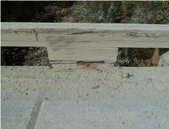
Figure 1-7: Typical guardrail condition.
