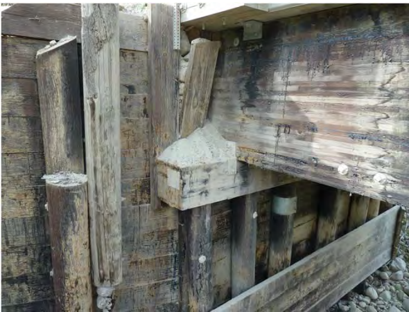
Figure 1-17: Camp end abutment downstream, note damaged ballast wall plank.
