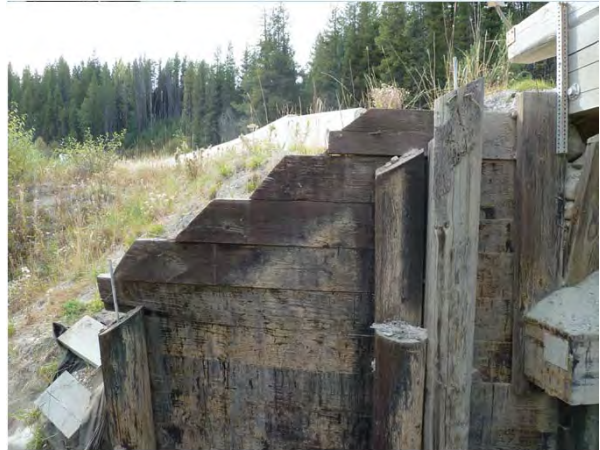
Figure 1-14: Downstream camp end wing wall, note missing top cap beam.
